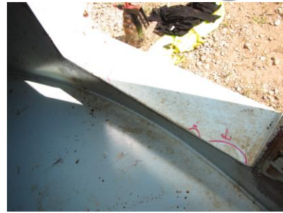
MANWAY COATING FAILURES
