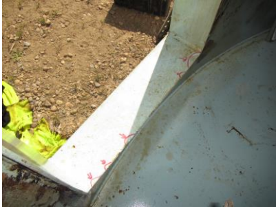
MANWAY COATING FAILURES
