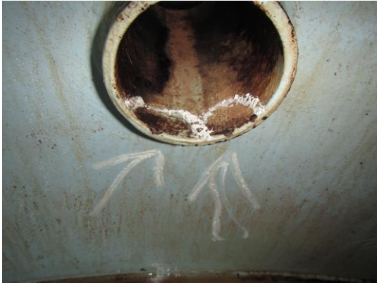
NOZZLE COATING FAILURE
