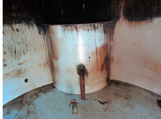
HEATER SECTION INTERNALLY
